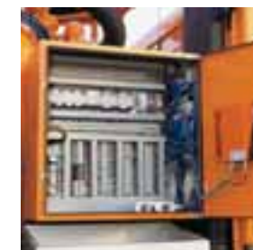
PLC, remote control, pneumatic and electric control placed centrally in a cabinet behind the driver's cabin. Eases possible faultfinding.
