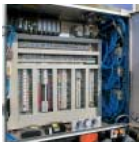
PLC, remote control, pneumatic and electric controls are gathered in one cabinet placed behind the cabin. This simplifies maintenance and faultfinding.
